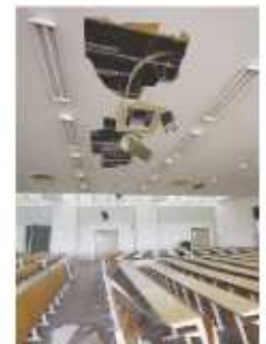
The ceiling of a classroom which collapsed by the earthquake.
